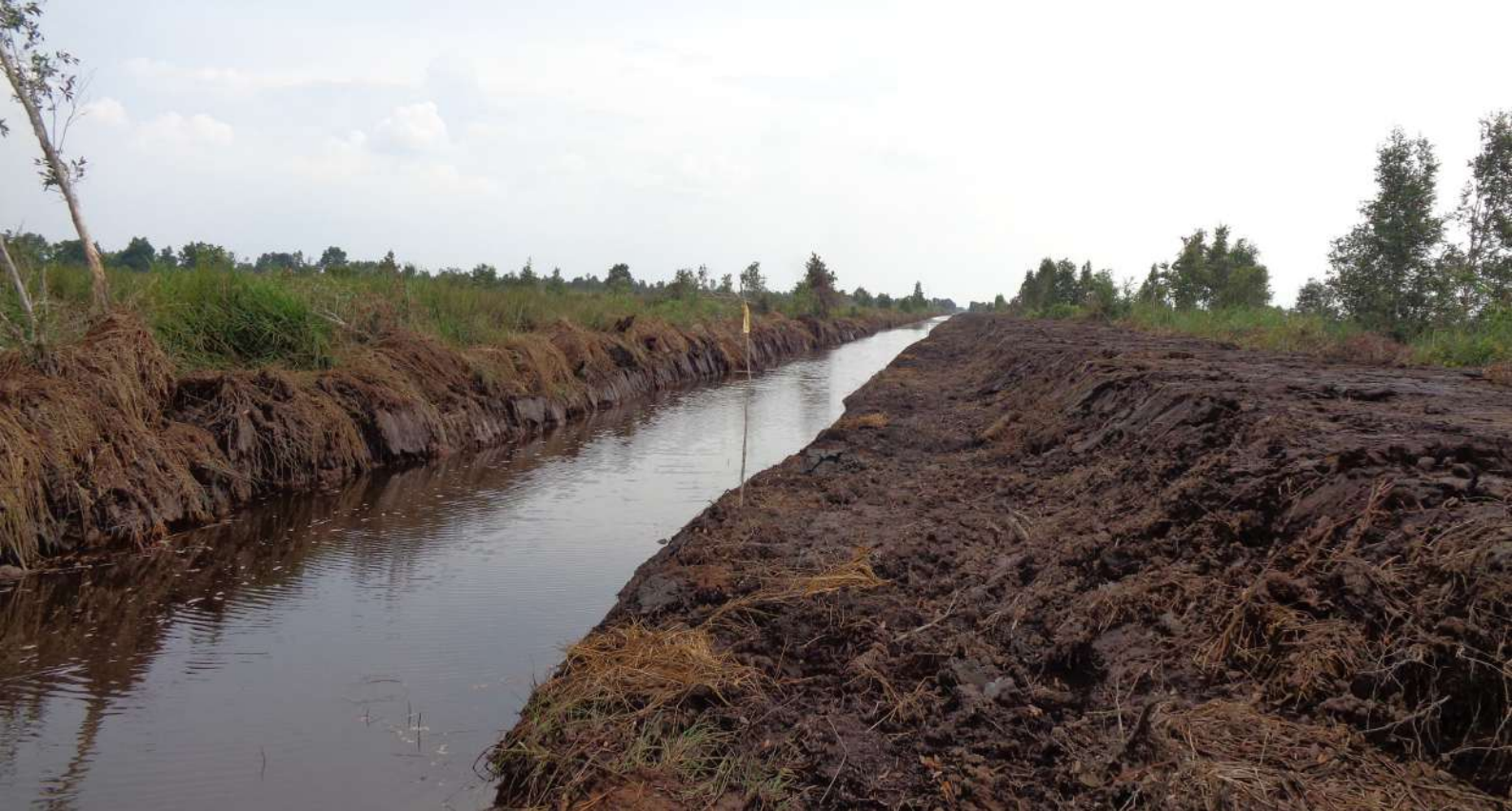
Gambar : Rehabilitasi dilakukan dengan memperluas dan memperdalam kanal sehingga meengeruk keluar tanah gambut. / The rehabilitation was implemented by expanding and deepening the canal which dug out the peat.
