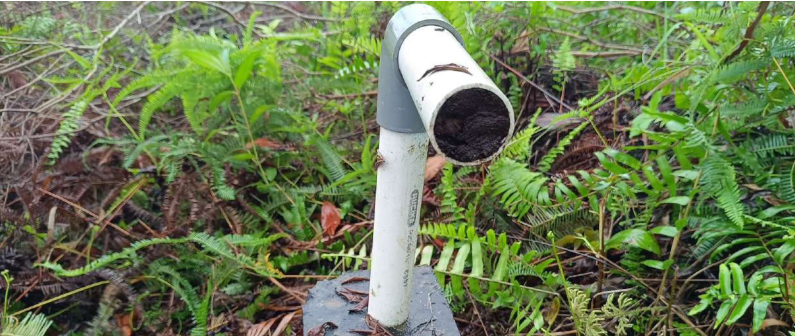
BRGM tube well pipe blocked by sediment in the Rokan ↑ River PHU, Riau Province. ©Pantau Gambut, 2024
