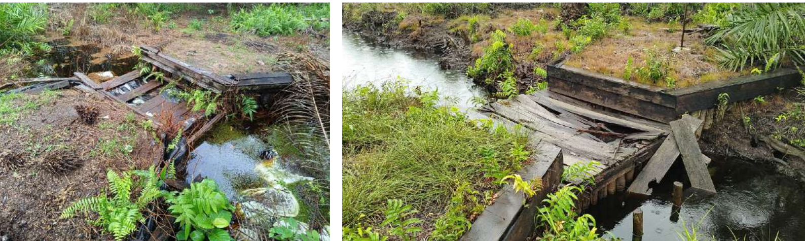
Damaged BRGM canal blocks found at (left) the Rupert Island KHG and (right) the Rokan River–Siak Kecil River KHG, Riau Province. ©Pantau Gambut 2024
