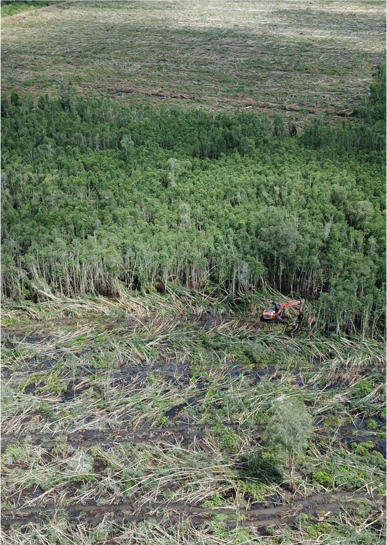
A land-clearing excavator at PT WUL's palm oil plantation site, located near the Food Estate expansion area in Tajepan Village, Kapuas Murung District, Central Kalimantan ©Pantau Gambut 2024
